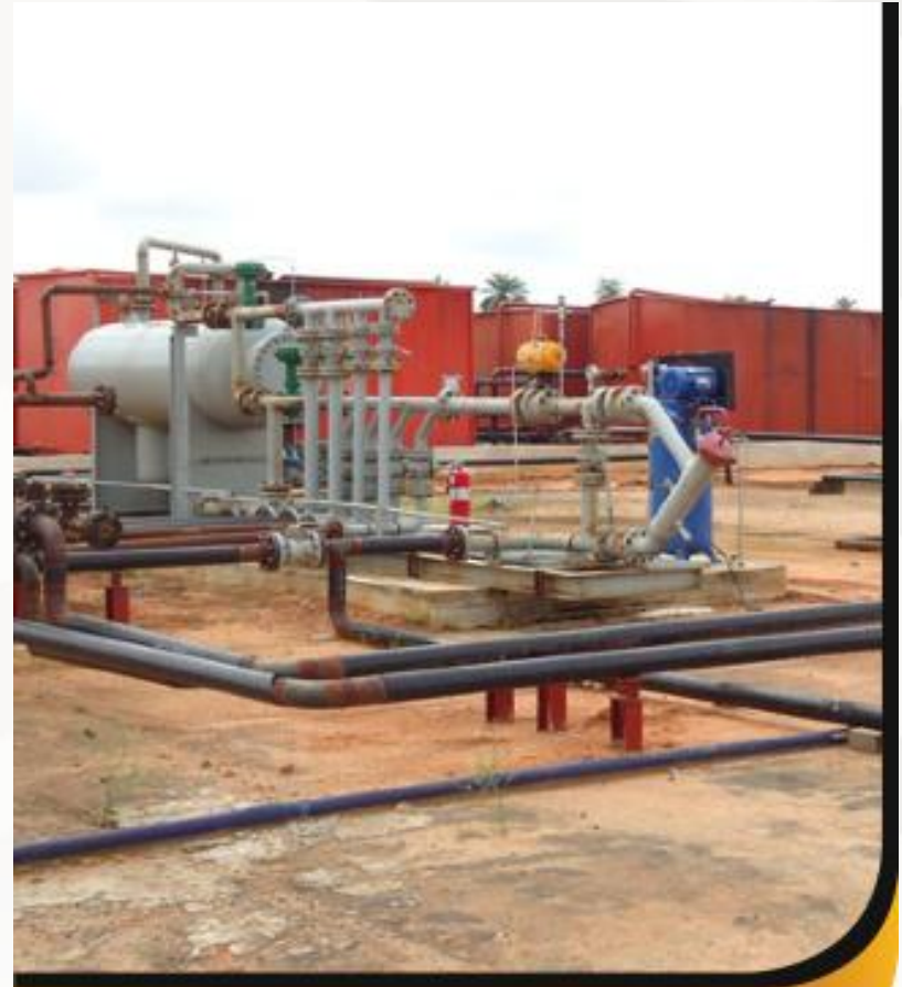
Early production equipment
